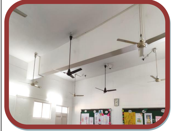
Ceiling Fans added in class rooms
